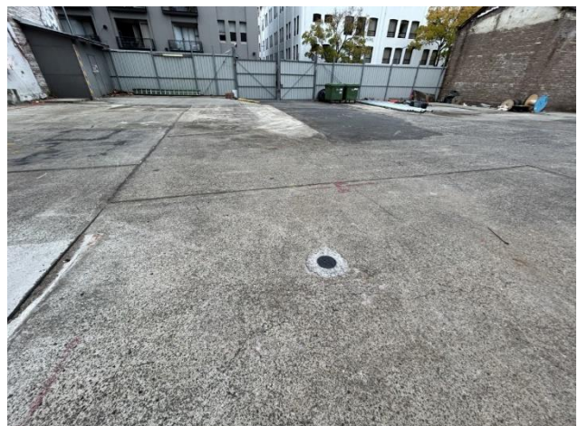
Figure 18 - View north detailing a ground monitoring well.
